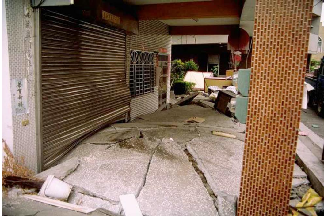
Figure 1-4. Punched footings and intermediate slab heaving due to cyclic softening of high-plasticity clay in Wufang, Taiwan. Photo by R. Seed (1999).
