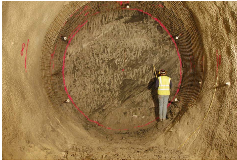
Figure 4-24. View of FE tunnel face from the FE niche showing beddings dipping 45^\circ (Viotor, 2012).
