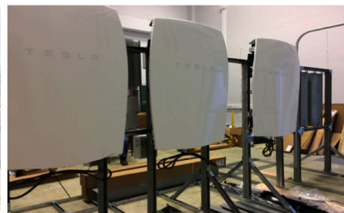
(b) 7.2 kWh local energy storage capacity with a peak output of 3.3 kW (only two of the three shown have been used in this experiment)
