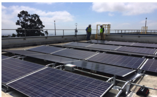
(a) 3.64 kW local solar power generation
