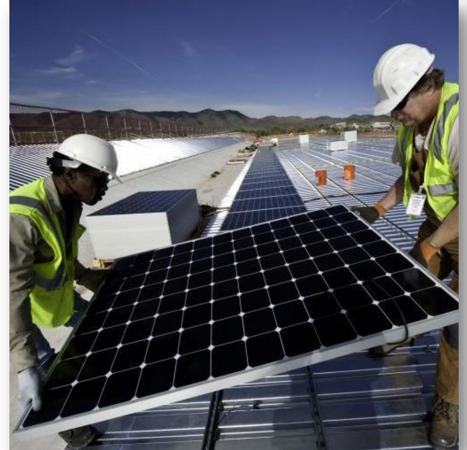
Photo c/o Department of Energy Solar Workforce Development
