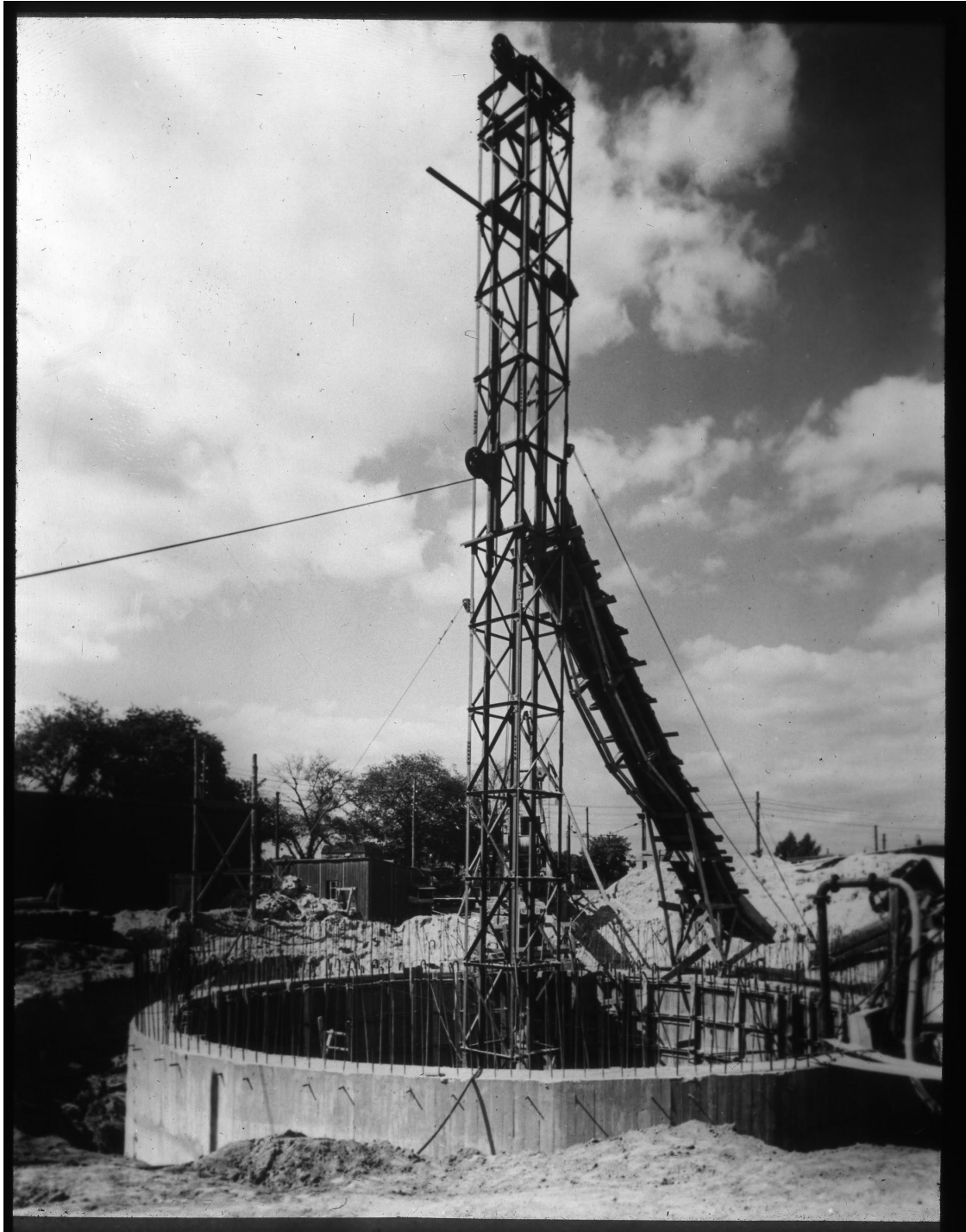
Fig. 27. Degebo. Air pressure pump designed to keep the water out of the pit during the digging work. 1941. Diaarchiv Degebo.
