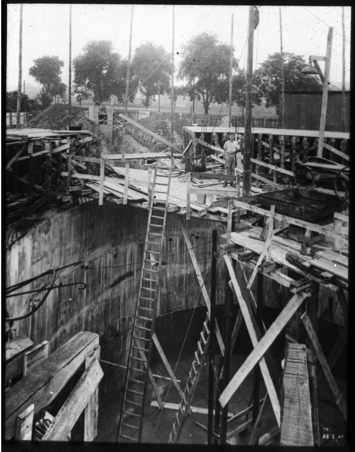
Fig. 76. Degebo. Pit of the heavy load-bearing cylinder in the early stages of construction. 1941.
