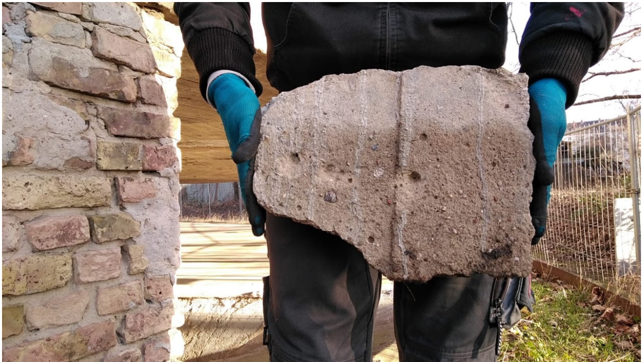
Fig. 44. Krüger, René. Chunk of concrete that fell off the cylinder. 2019. Jpeg.
