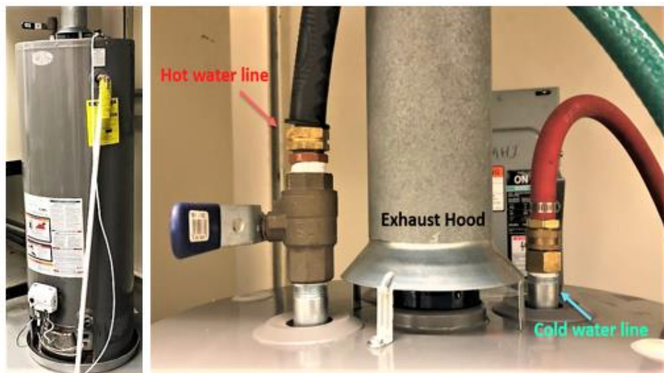
Figure 24. Gas storage water heater and pipeline connection
