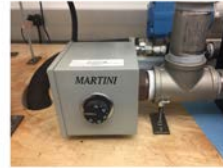
Figure 3.3.8.1: Heater for varnish test system with specifications.
