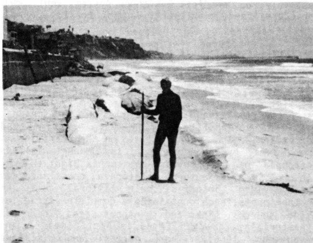
Figure 1. Longard Tube installation at San Clemente, California. Photo taken in May 1982. Note, a total of three tubes have been installed parallel to each other in some places. Photo G. Kuhn.
