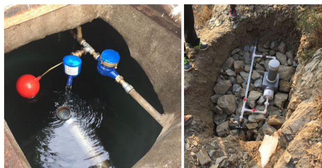
Figure 1. (Left) Aquatabs Flo technology installed at the inlet to a reservoir tank. Pretreatment samples were collected from the unchlorinated bypass. (Right) PurAll 100 technology installed in-line just upstream of a reservoir tank. Pretreatment samples were collected from a sampling tap, visible just upstream of the device.
