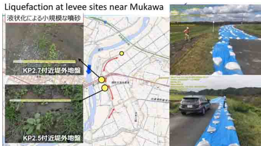
Figure 5.8: Sand boils observed by Japanese researchers (left). Blue tarps on top of the flood control levee (right). (photos taken by the GEER field reconnaissance team [42])
