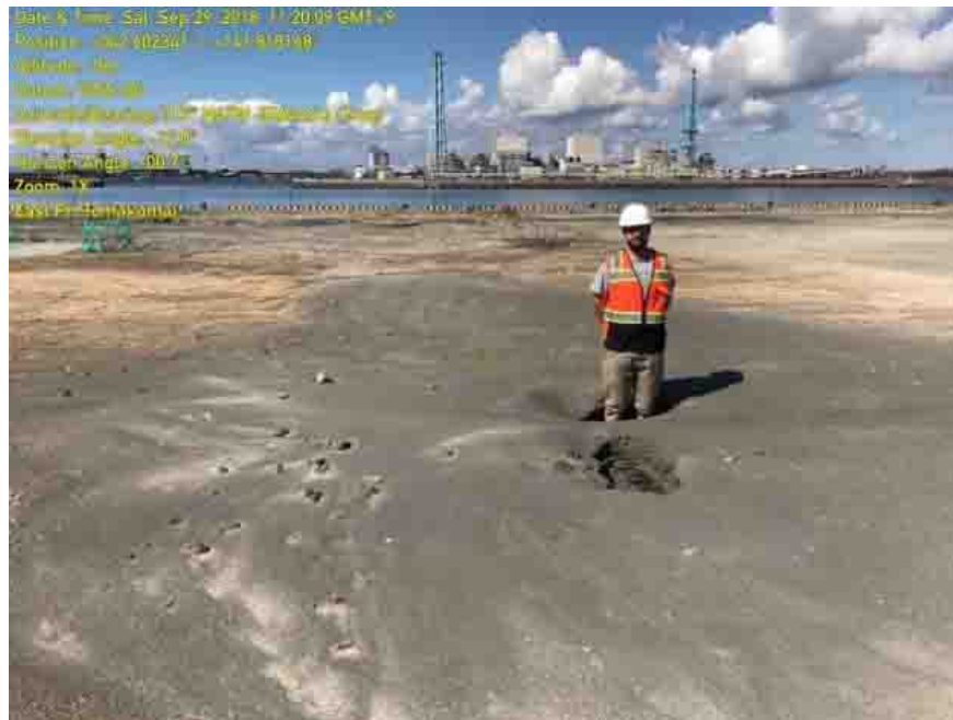
Figure 5.6: Sand boils in an undeveloped area where Tomato-Atsuma Thermal Electric Power Plant is in sight (photo taken by the GEER field reconnaissance team [42])
