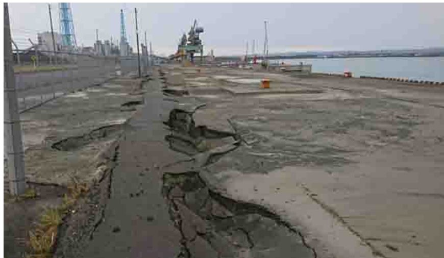
Figure 5.4: Uneven subsidence of road due to liquefaction with sand boiling in Tomakomai (photo taken by Watabe, Y., Hokkaido Univ.)
