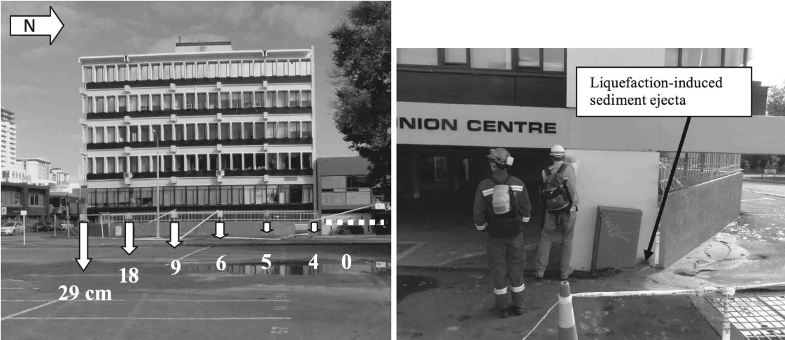
Figure 3.23: Building undergoing significant liquefaction-induced differential settlement due to part of it being founded on the liquefaction feature in this area (24 March 2011; S43.52878 E172.64252) [15].
