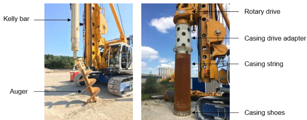
Figure 1: Rotary drilling rig at test site of Bauer Group in Schrobenhausen, Germany (Pictures by Fischer, A.)
