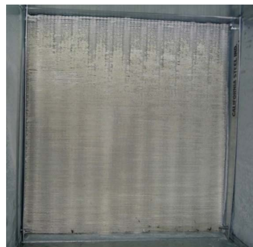
FIGURE 1 - EXAMPLE HEAT EXCHANGER AT FAILURE
