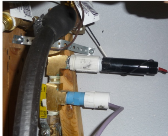
FIGURE 8– PH AND CONDUCTIVITY SENSORS IN WATER LINE OF SPRAY WATER
