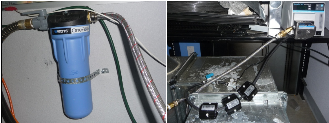
FIGURE 5 - INSTALLATION OF ONEFLOW (LEFT) AND GMX WATER TREATMENT (RIGHT)
