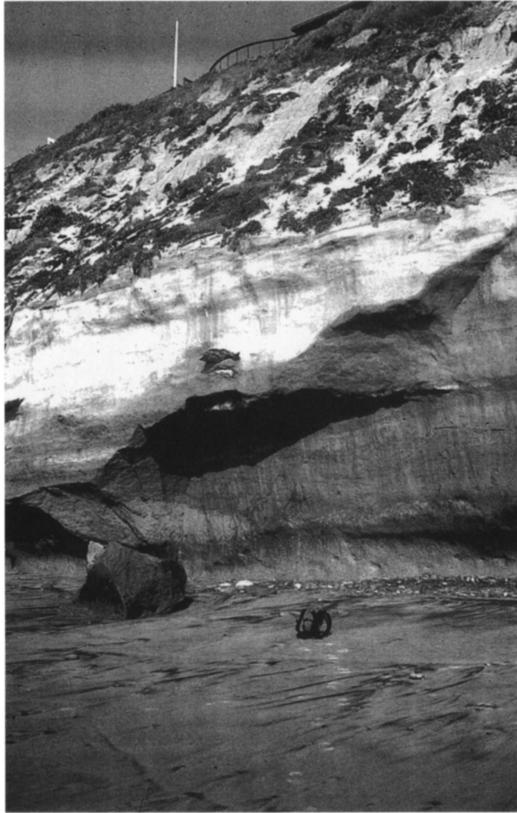
Figure 2. Block quarrying of jointed sandstone at the Solana Beach site. These cliffs are frequently attacked by waves regardless of tidal height.
