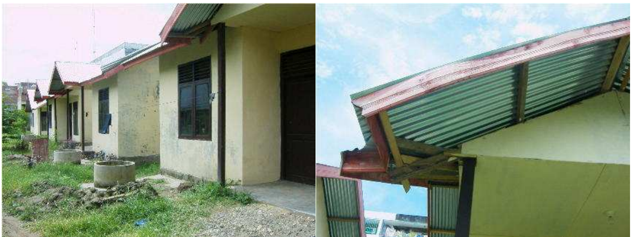
Figure 5.2: A house built by BRR that deteriorated before occupancy
