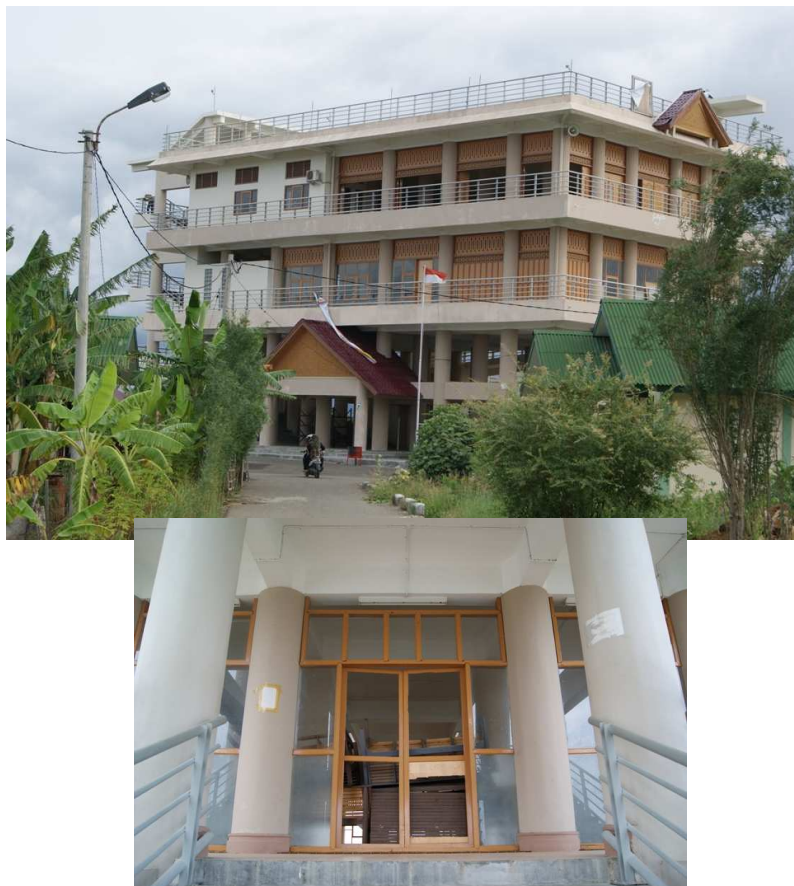
Figure 6.2: One of three escape buildings in Banda Aceh had deteriorated in many places due to lack of maintenance
