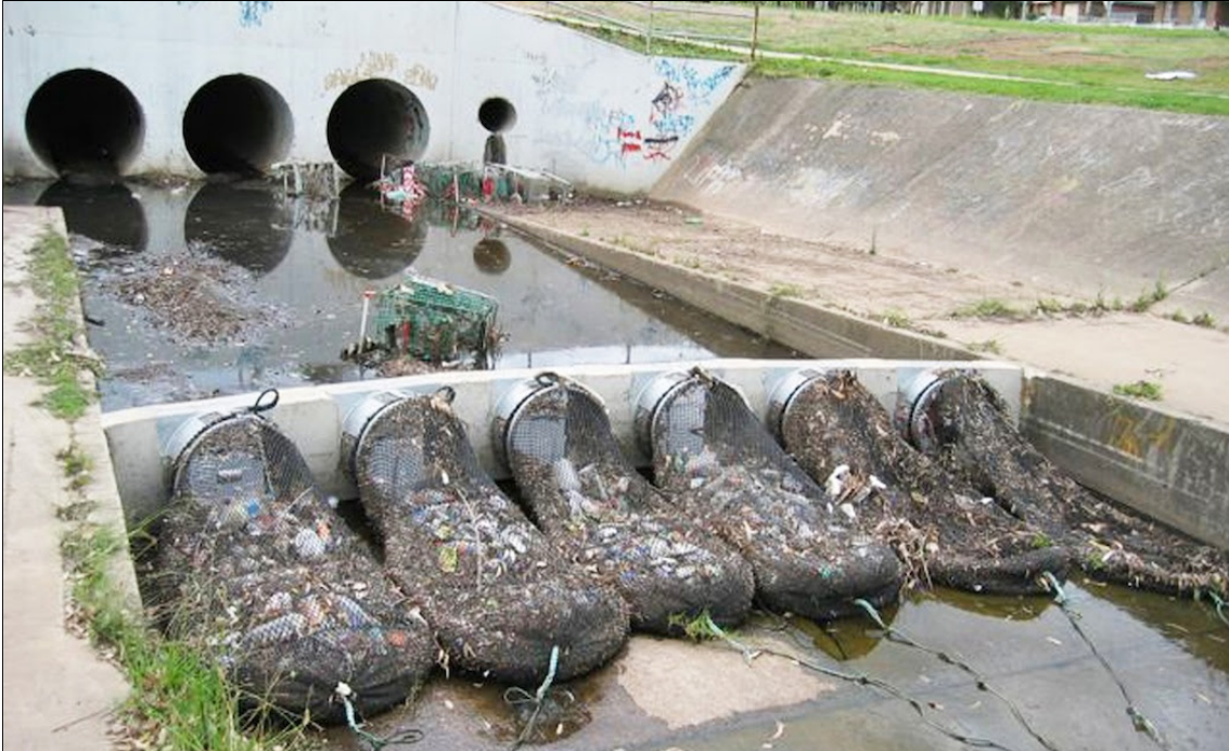
An example of a system of nets for capturing trash in creeks and storm drain channels.
