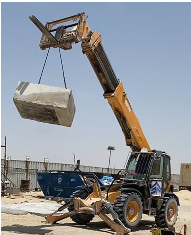
Figure 13. Impact load generation by a concrete mass.
