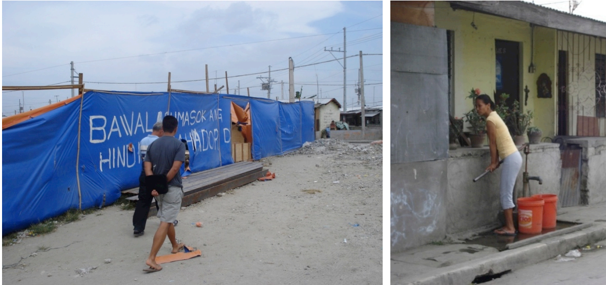
Figure 3.1. Marilou’s micro-network project in Biñan. To the left, a cordoned-off area where she is installing a deep well. To the right, the shallow handpumps that the NHA supplied. Photos by author.
