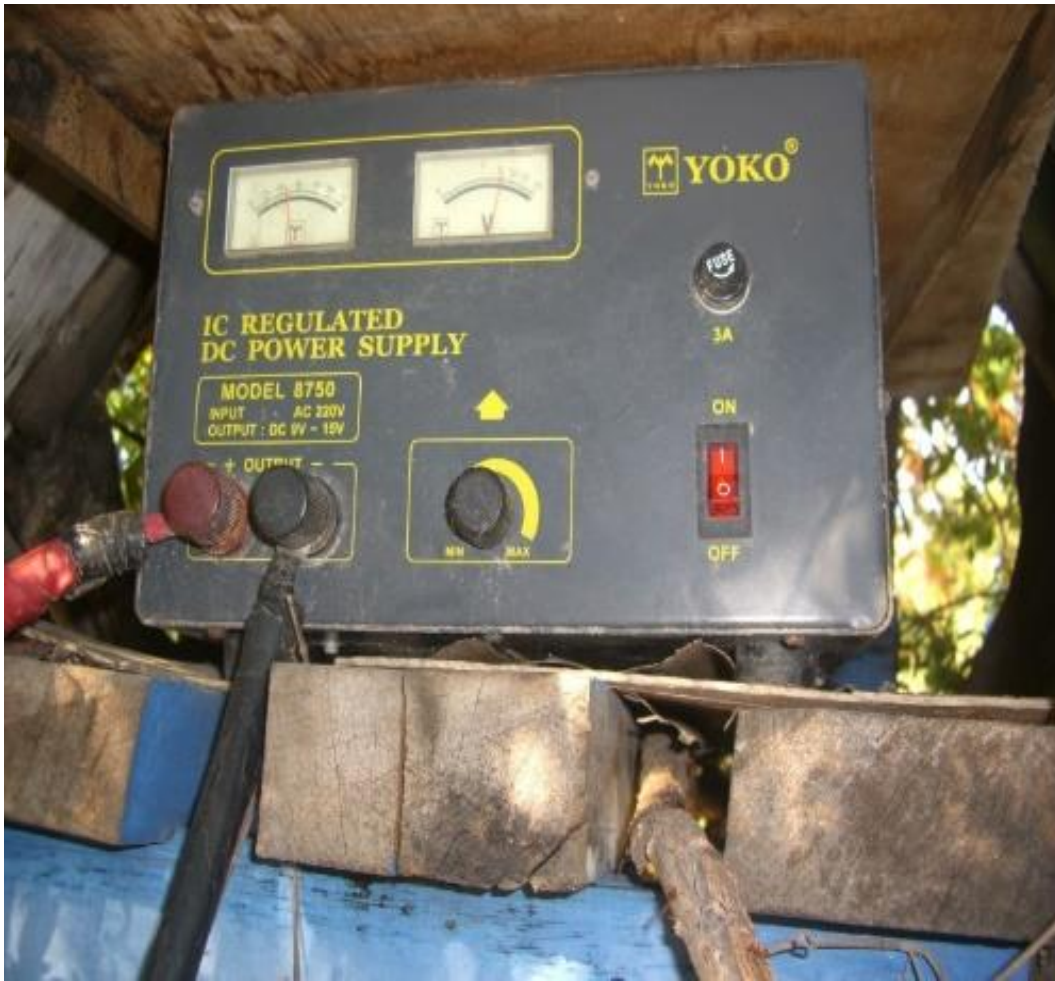
Figure 4. DC power supply with output cables leading to a Biorock installation in Indonesia. Note current and voltage output meters.
