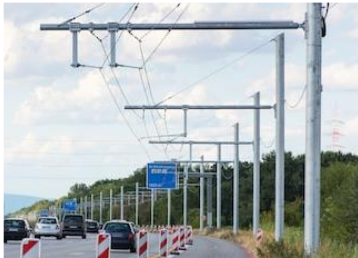
Figure 8. The eHighway contact line. A specially designed two-pole contact-tine system ensures a secure energy supply to the trucks [48].
