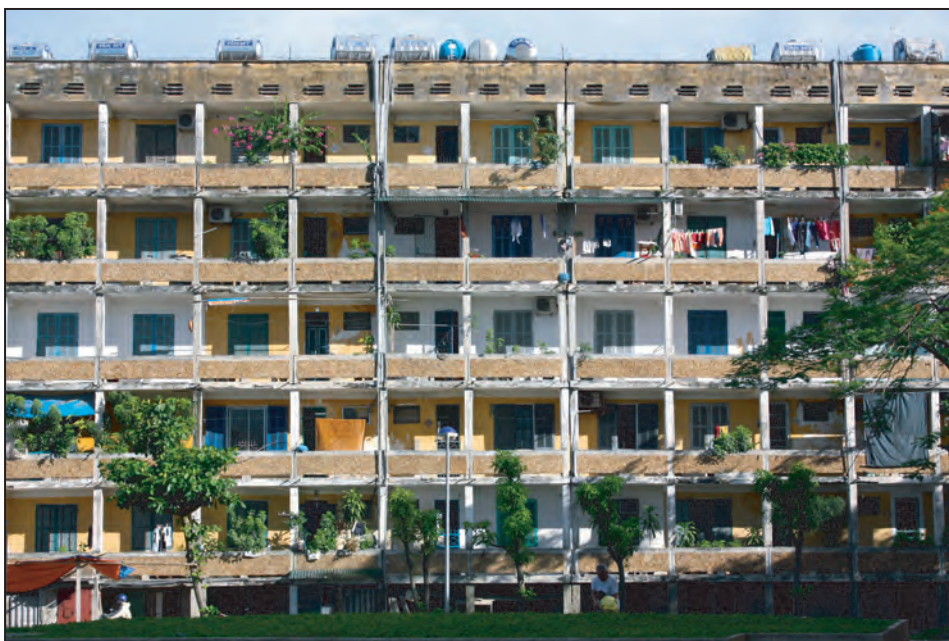
Figure 3. Open row design of Quang Trung to facilitate natural lighting and air flow (contrast with interior-oriented design in Figure 1), 2010. Photo by the author.
