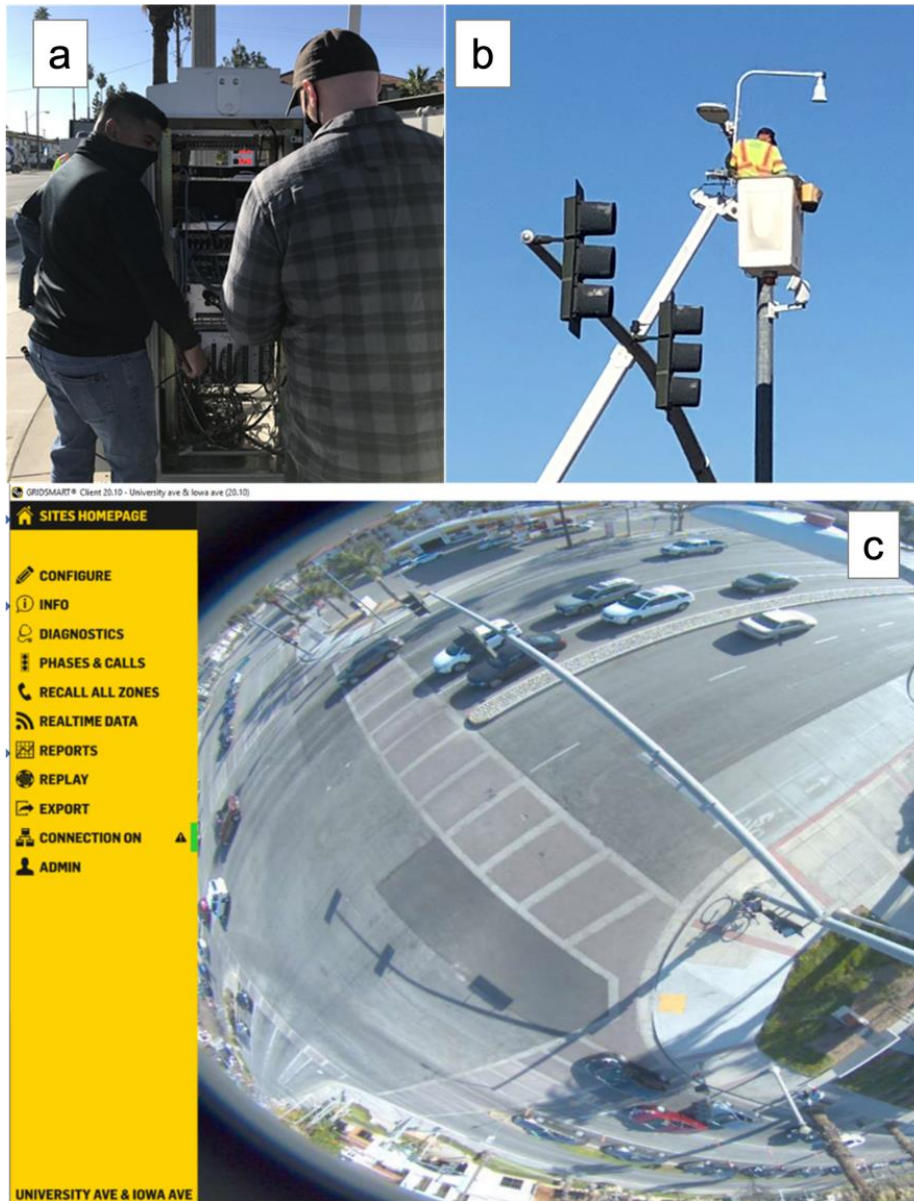
Figure 2. Installation and user interface of GridSmart Fisheye Cameras. a) Researchers at the traffic controller cabinet. b) Installing the camera on a streetlamp post. c) GridSmart user interface.
