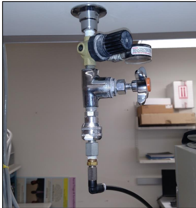
Figure 42: Image of Building Air Compressor
