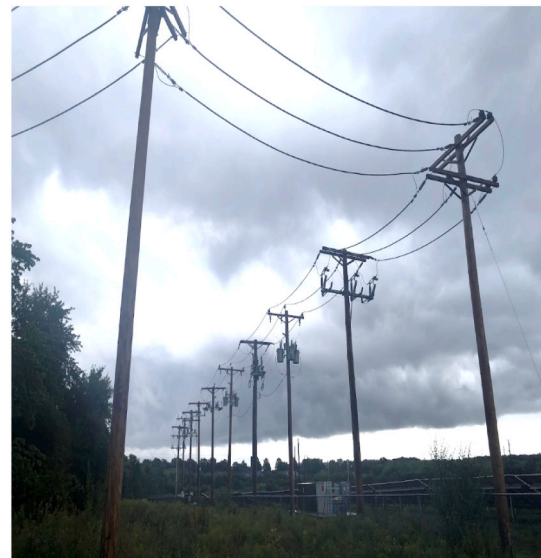
Photo 2. Visual impact of interconnection infrastructure.
