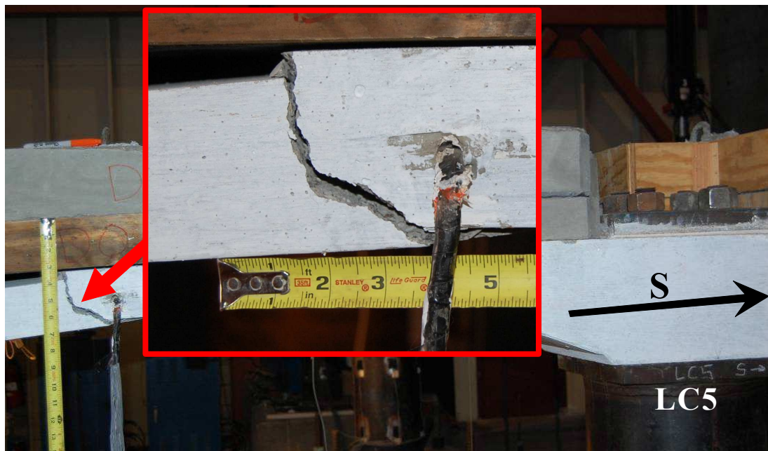
Figure 4.27: Localized failure near LC5 during test at slab-slab corner.
