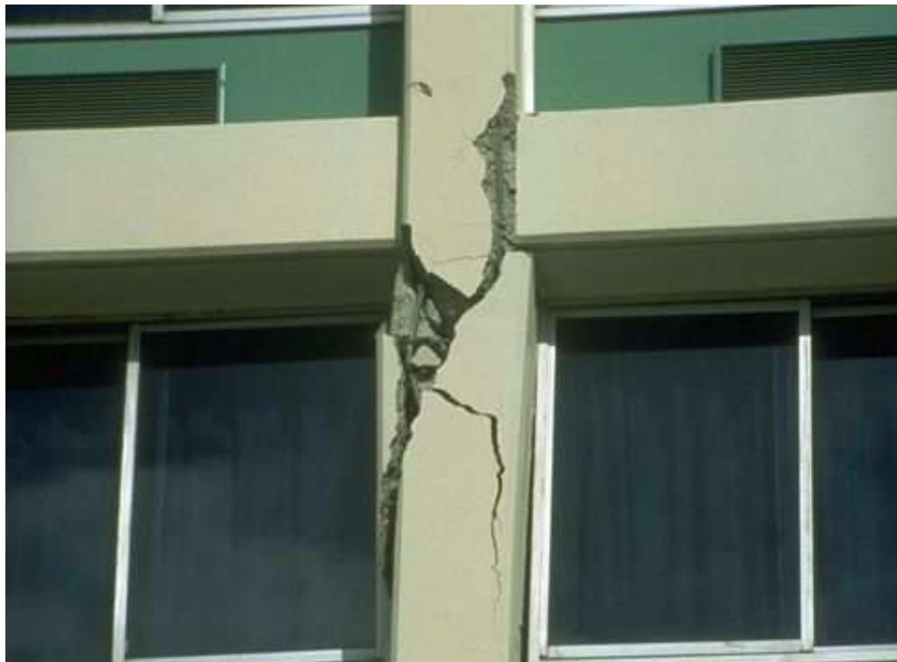
Figure 1.4: Shear failure in columns at the Van Nuys Holiday Inn during the 1994 Northridge earthquake, 1994; (photo courtesy: Peter W. Clark)
