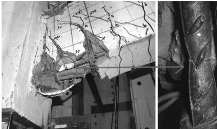
Figure 2.1: Rebar rupture at bottom of the beam next to the joint where column was removed (from Yi et al. 2008).
