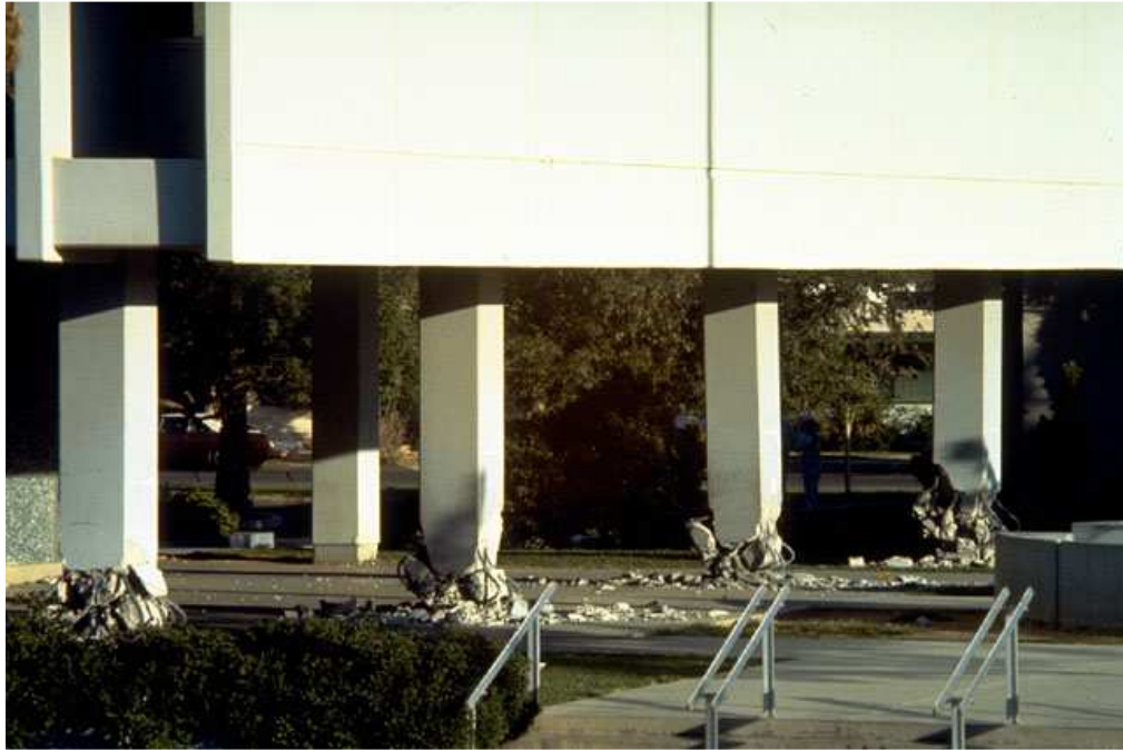
Figure 1.3: Shear failure of columns at the Imperial County Services Building during the Imperial Valley earthquake, 1979 (photo courtesy: Vitelmo V Bertero).
