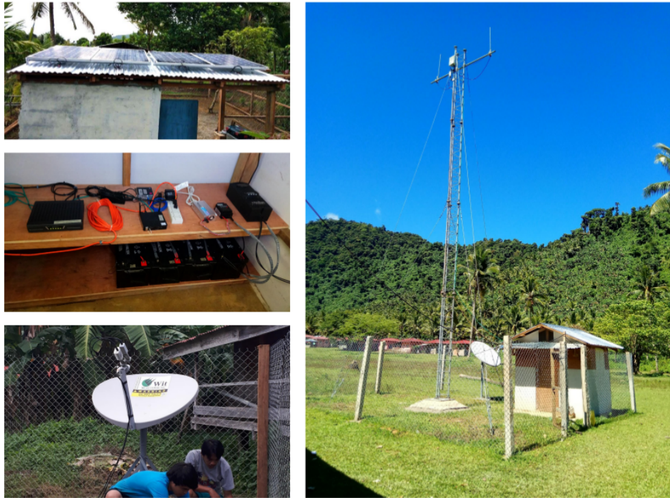
Figure 4.5: Components of a typical UP community cellular installation: solar panels (top left), battery bank and network hardware (middle left), VSAT antenna (bottom left), outdoor GSM radio system, tower and shelter (right).
