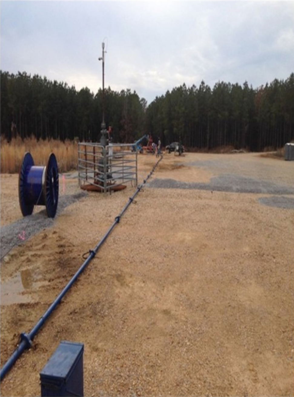
Fig. 4. Flow iron looking toward F1 well from F3 well. This is the main recirculation loop for geothermally heated CO 2 . The F2 well head appears in the foreground with the more distant F1 well head painted red beyond it.
