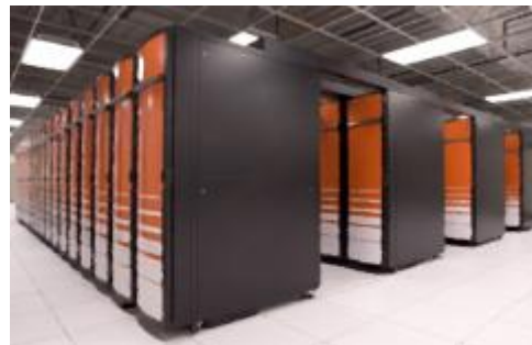
Figure 18: Data Center Using Advanced Cooling Controls
