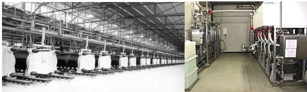
Figure 3: 135 MW KOH electrolyzer plant on left and 1 MW PEM system on right
