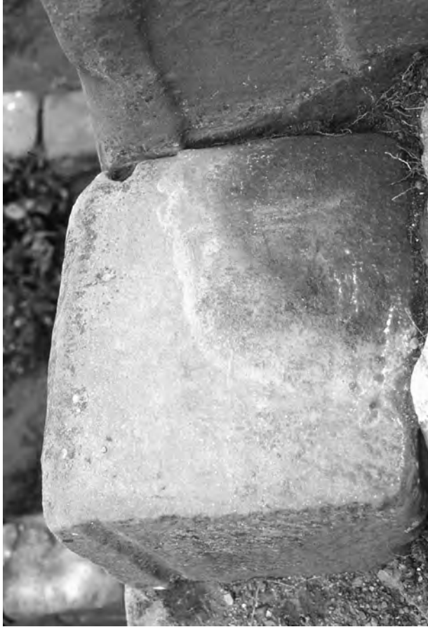
Figure 6.22. Rabbet joint on upright. Also note the rope chase on the block fitted to upright.
