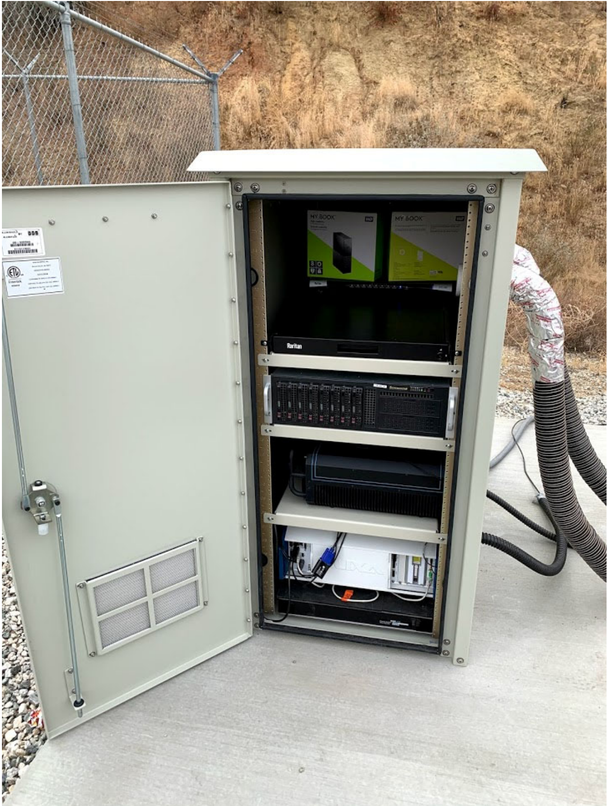
Figure 2-2. Picture of instrumentation rack
