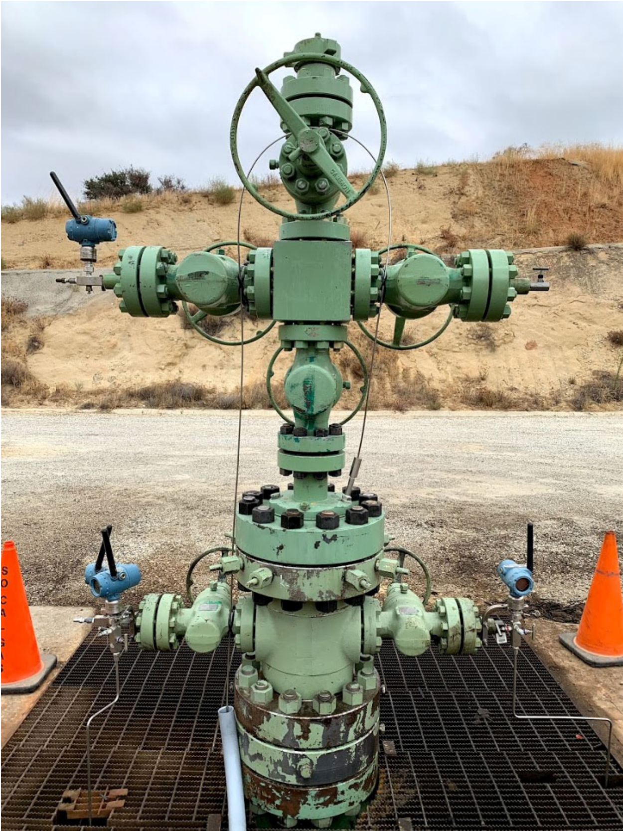
Figure 2-5. Picture Showing the Hydrbid cable in Figure 2-4 connected to the wellhead
