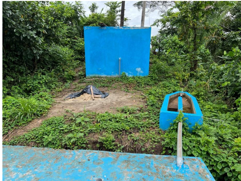
Figure 13. This water storage tank at Llucanayacu was built during the 2010s as the first phase of the water distribution system. In 2022 the community was working to connect it to a plumbing system to distribute water to the community's schools. Photos taken by author March 28, 2022.
