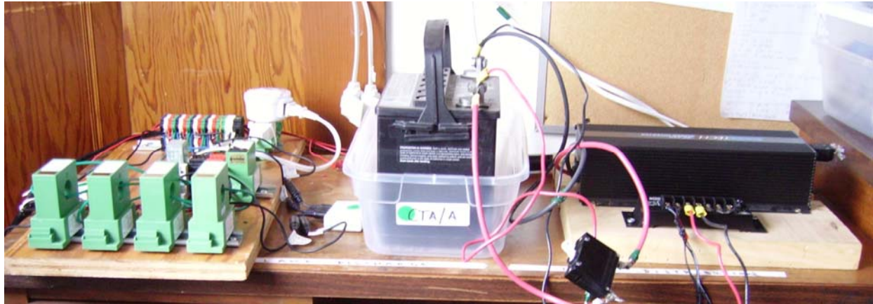
Figure 7. AC Power Supply for Grid Charging. 230V/50Hz pure sine wave inverter (far right), 6 V battery to power the inverter (middle), datalogging equipment (far left).
