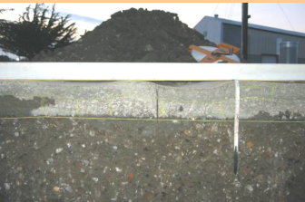
Test pit profile, note rutting in lower AC layer
