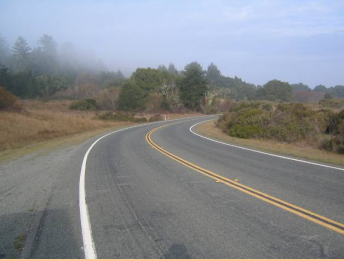
Consistent bleeding/stone loss
