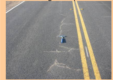
Pumping through crack
