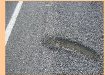
Raveling on chip seal
