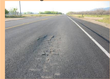
Fatigue crack, base failure
