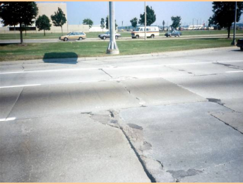
Inconsistent concrete surface
