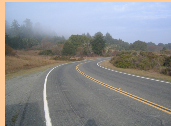
Failed chip seal (>20% stone loss)
