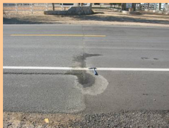
Patch joint failure
