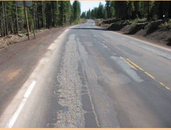
Inconsistent rutting and cracking
