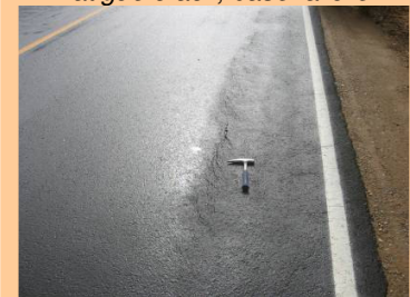
Shear crack, base failure
