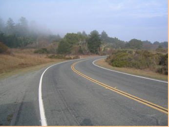
Consistent bleeding/stone loss
