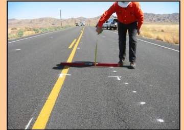
Visual assessment of rutting
