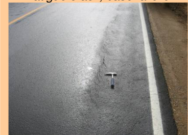
Shear crack, base failure
