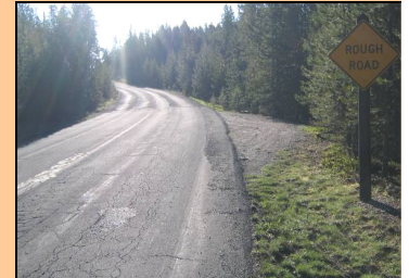
Road is curved, sight distance is limited, and structure is inconsistent.
