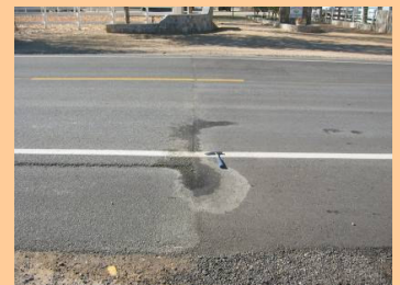
Patch joint failure
