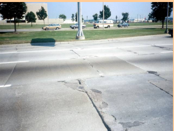
Inconsistent concrete surface
