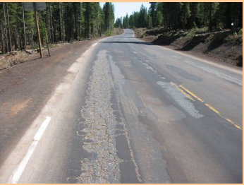
Inconsistent rutting and cracking
