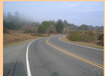
Failed chip seal (>20% stone loss)
