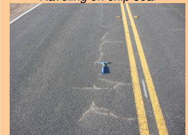
Pumping through crack
