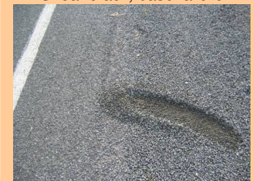
Raveling on chip seal
