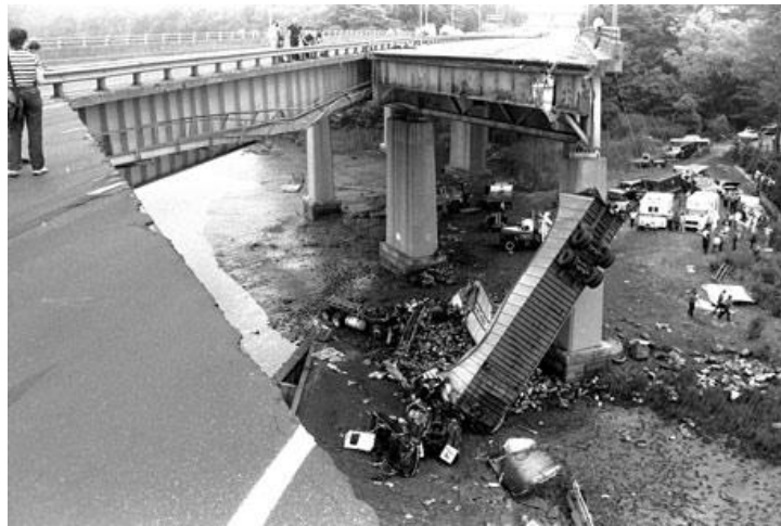
Fig. 1.1: Bridge: Mianus River Bridge in Greenwich, Conn. | Disaster: Structural failure caused the bridge to collapse, and vehicles plunged into gap | Fatalities: 3 |
