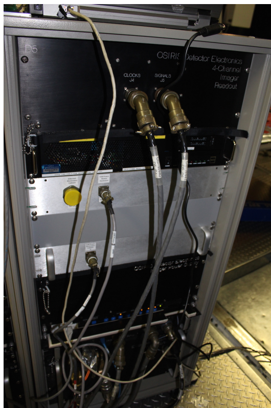
Figure 3.5: An image of the electronics rack that contains the new detector control computer and the SAM power supply enclosure. A computer interface panel holds the USB and Gigabit-ethernet mil connectors that connect to the control computer. All of the H2 power and readout electronics have been removed and replaced by the new H2RG components. This electronics rack still contains the original imager detector electronics, which will be replaced in the future as a part of the imager upgrade project.
