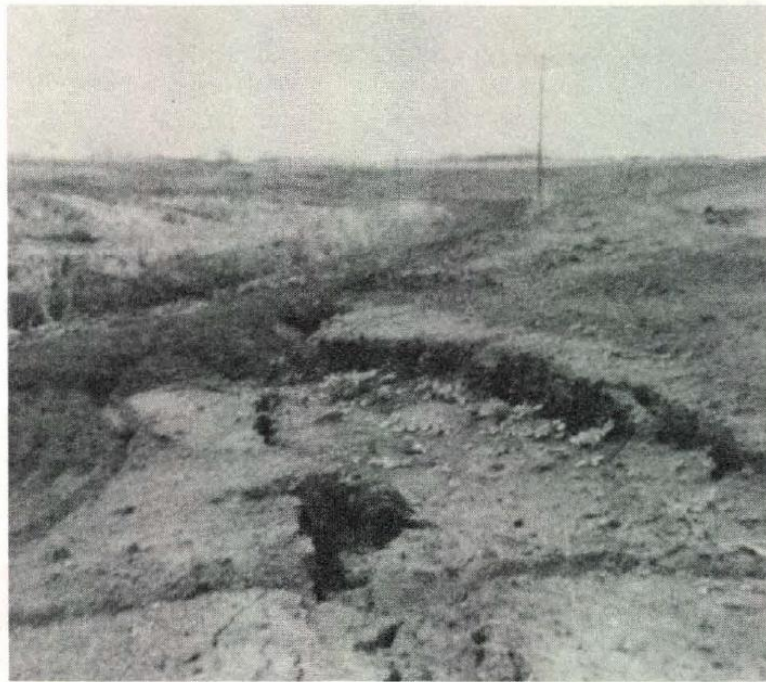
Levee damage on Bacon Island (Site 2). A 250-foot land-side rotational slip-out dropped several feet during the January 24, 1980 Livermore earthquake.
