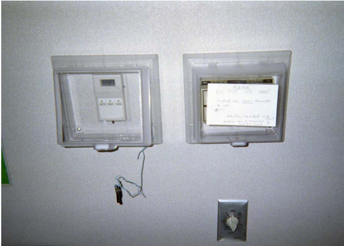
Figure 5: Side-by-side control thermostats for IDEC and standard HVAC systems in each field study RC. Plastic lock boxes and notes were used to remind teachers which system to use during the school year, given the case-crossover study design.
