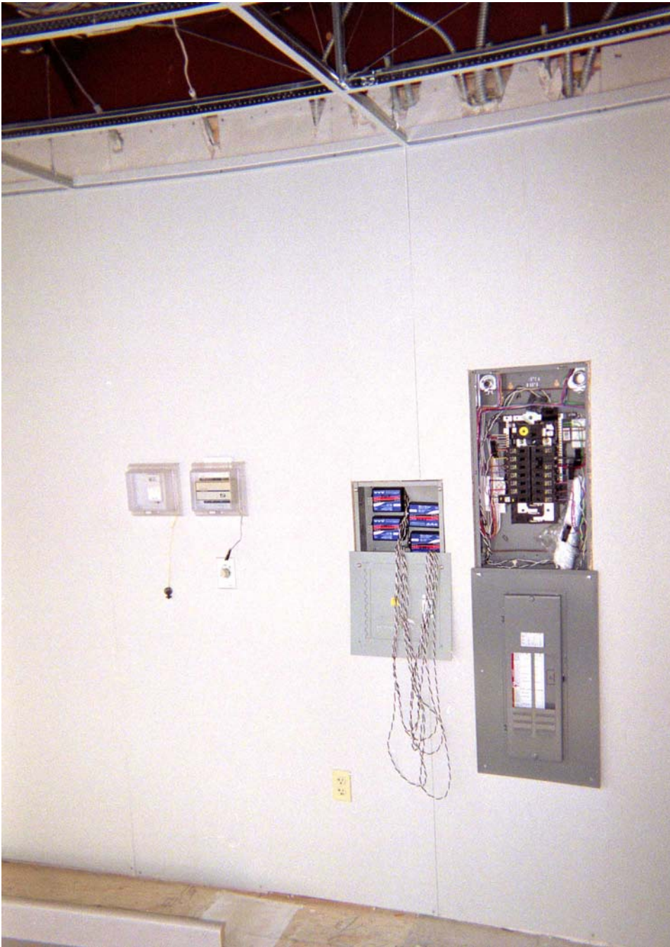
Figure 10: Photograph of P-Series WattNode digital pulse sensors (50A CT and 15A CT type), concealed in an electrical panel, used in each of the four RCs to measure total building (watt0), conventional HVAC heat pump (watt1), IDEC (watt2), and lighting (watt3) power for the electricity monitoring component of the field study.
