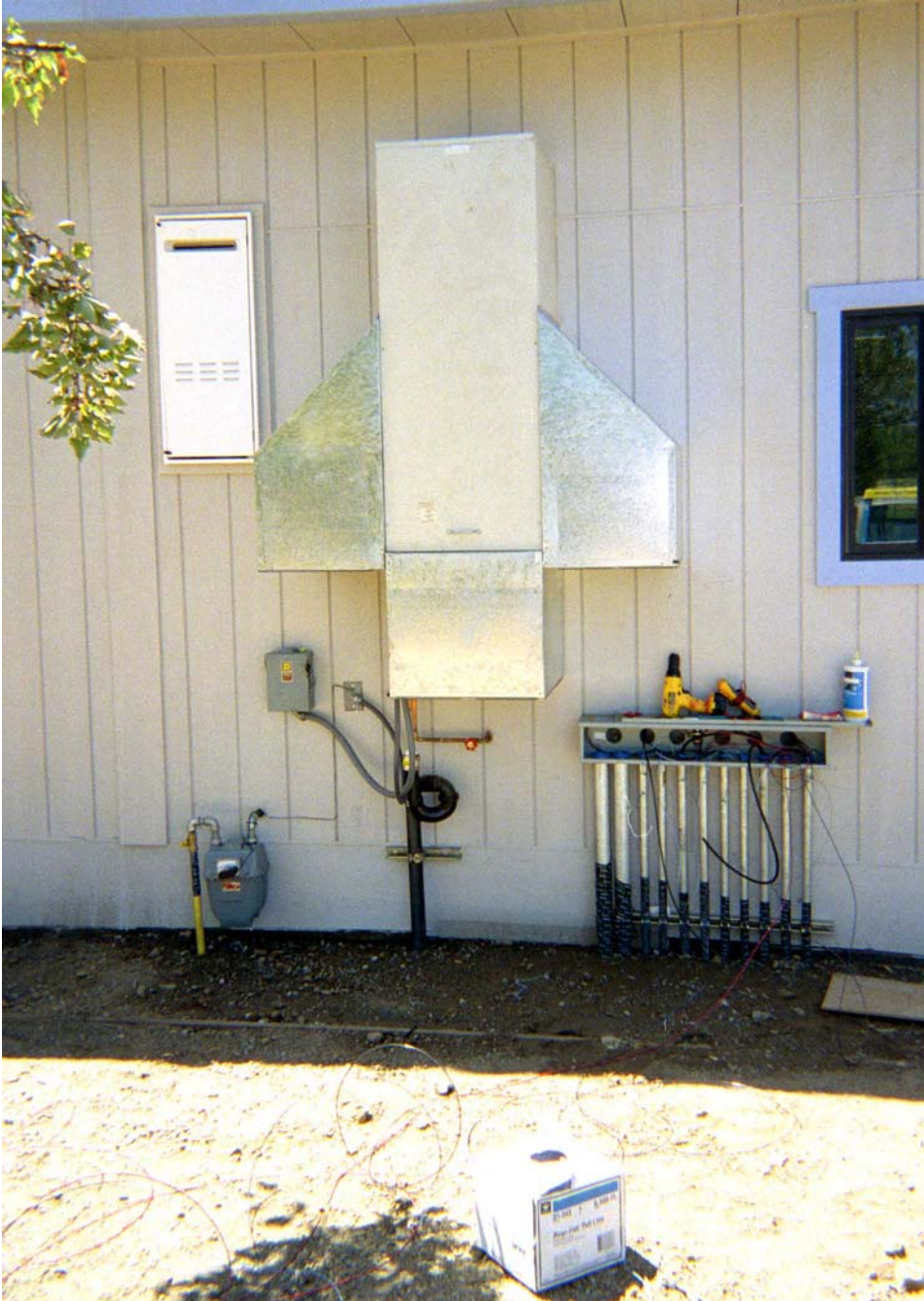
Figure 4: Photograph of the IDEC with LBNL customized inlet filtration system (65% ASHRAE dust spot efficiency DuraMax filters, two DM-603 and one DM-602, Koch Filter Corporation, Louisville, KY) mounted on the back wall of each RC.
