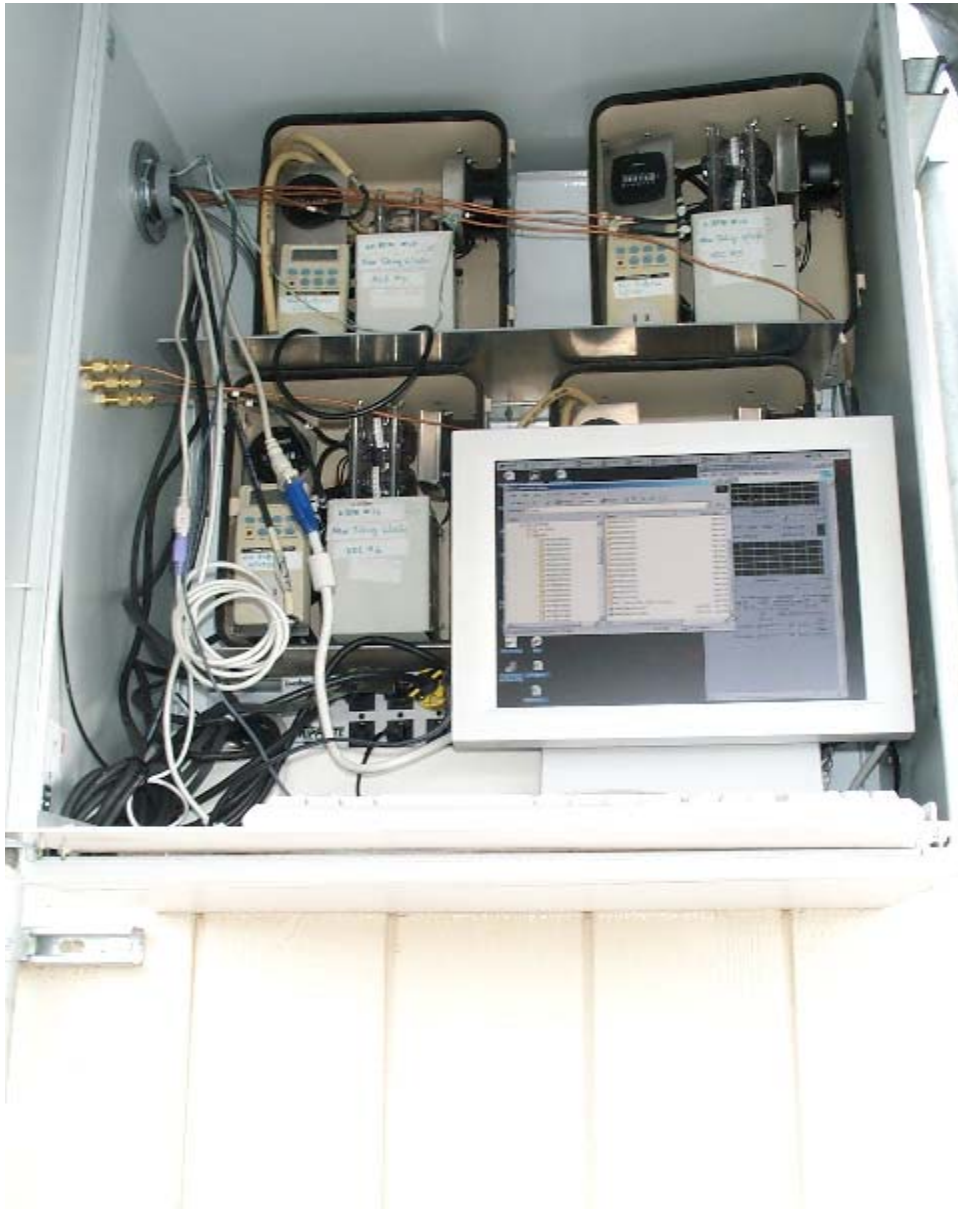
Figure 8b: Photographs of the completed (b) LBNL modified white, waterproof steel outdoor enclosure (Hoffman, Inc., San Francisco, CA) for environment monitoring and computer equipment.
