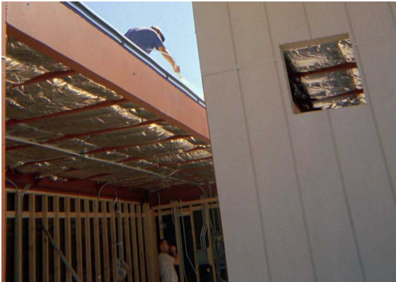
Figure 2 (a-b): Photographs of the application of the white paint “cool roof” provided for the four HPCBS Element 6 RCs.
