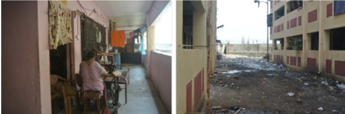
Figure 16: Built environment characteristics of location 1 (L1) a) Corridors treated as extended living spaces b) poor maintenance of common areas (Source: Authors).
