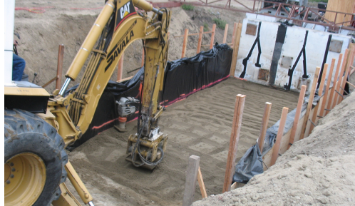
(b) Excavation of native soil to be substituted with the engineered backfill, UCLA experiment.
