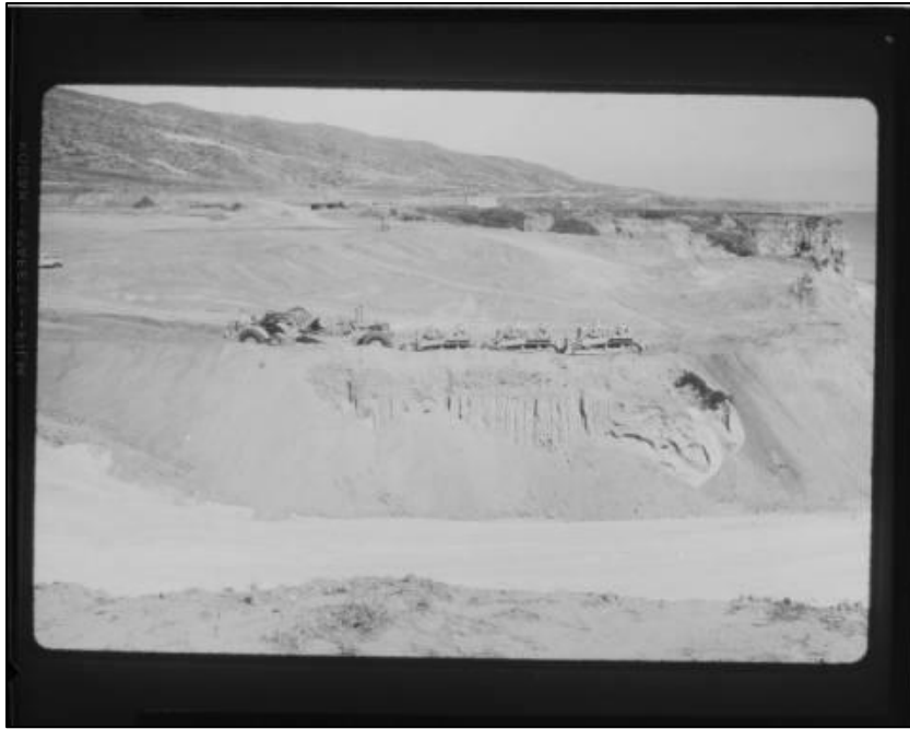
Photograph 1.9: A bluff is leveled to house the controversial San Onofre Nuclear Generating Station, which began operating on June 17, 1967 and shut down permanently on June 7, 2013, only ten days shy of its 46th anniversary.
