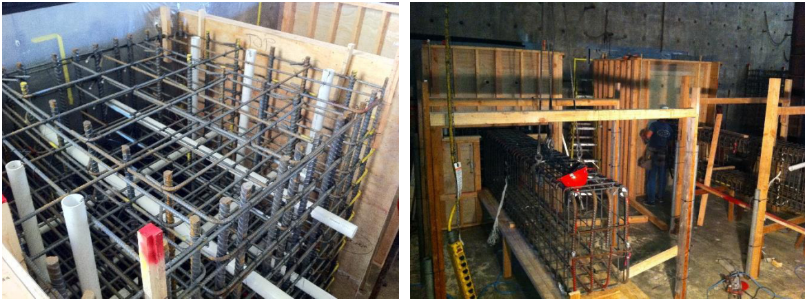
Figure 4.5: Left: Top view of reaction block for S1 reinforcement with PVC pipes into strong wall and strong floor; Right: Completed reaction block formwork and construction of beam formwork
