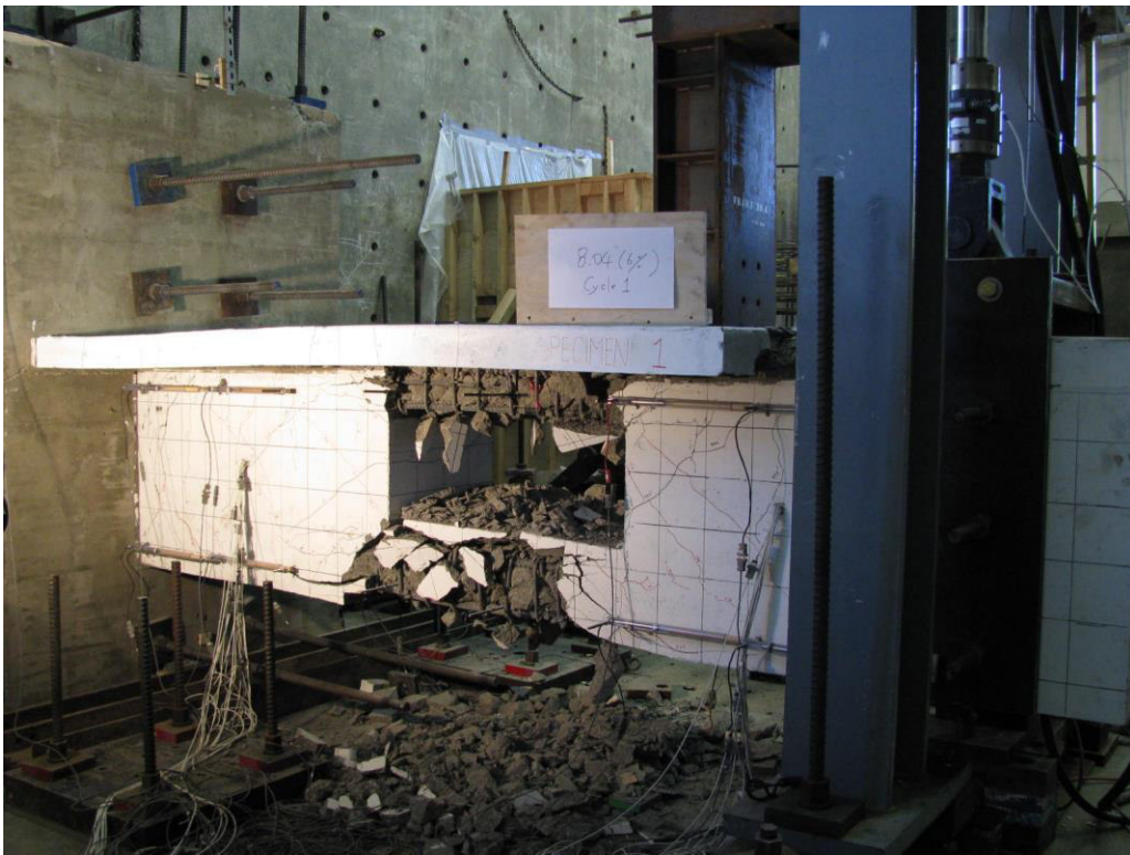
Figure 5.5: Crack pattern at 6.0% drift for S1
