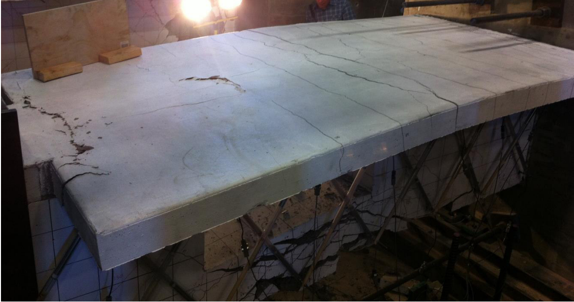
Figure 5.8: Cracking pattern on top of slab of S1
