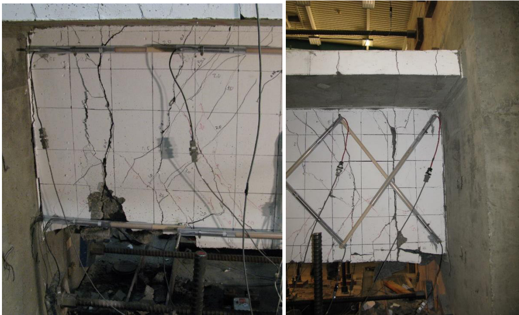
Figure 5.21: Cracking pattern at the fixed end at 3.0% drift on both sides of beam
