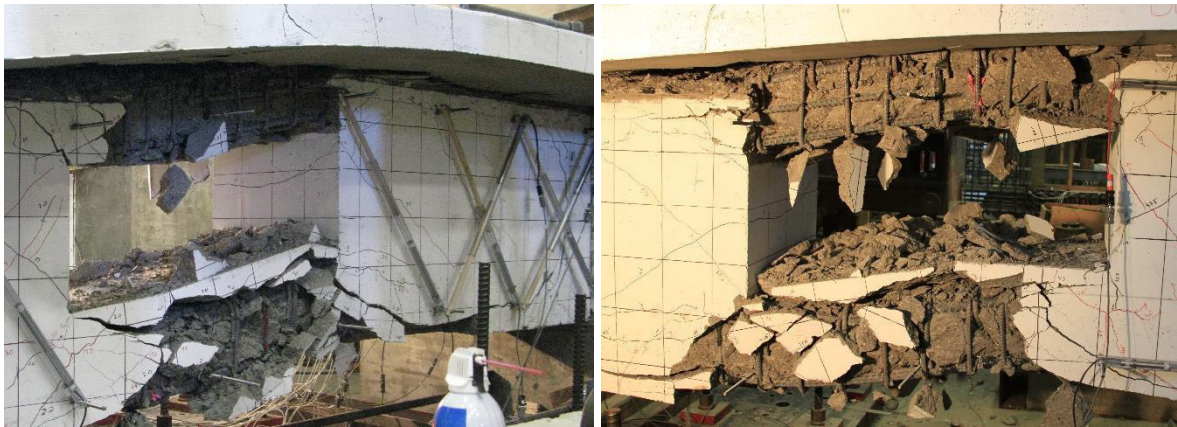
Figure 5.7: View of opening region on both sides of beam during 6.0% drift
