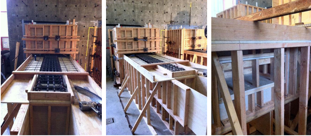
Figure 4.7: Left: Completed formwork for S1 and view of top slab reinforcement; Middle: Lateral formwork bracing; Right: Formwork around opening of S1
