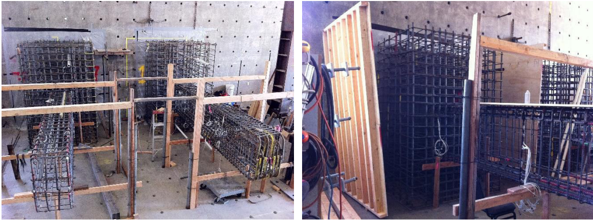
Figure 4.4: Left: Completed rebar cages for S4(left) and S1(right); Right: Formwork panels for the reaction block
