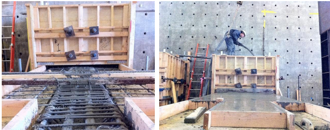
Figure 4.9: Left: Completion of concrete placement stage 1 (beam and bottom block) of S1; Right: Top slab for S1 is completely poured; Pumper fills up the top of the reaction block
