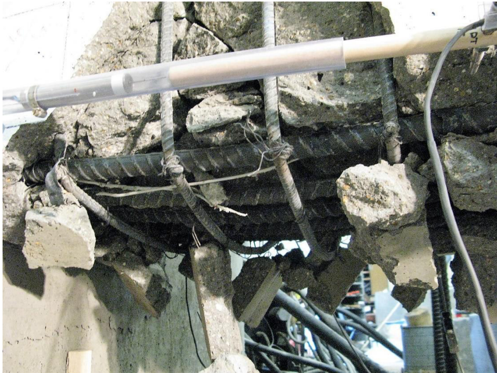
Figure 5.23: Exposed bottom longitudinal reinforcement at end of test for S3
