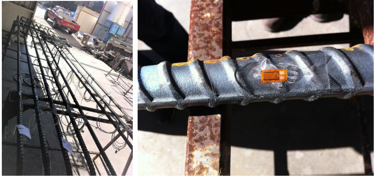
Figure 4.19: Left: Strain gauges installed along the longitudinal rebar before cage construction; Right: Strain gauge attached to a #8 bar during installation process
