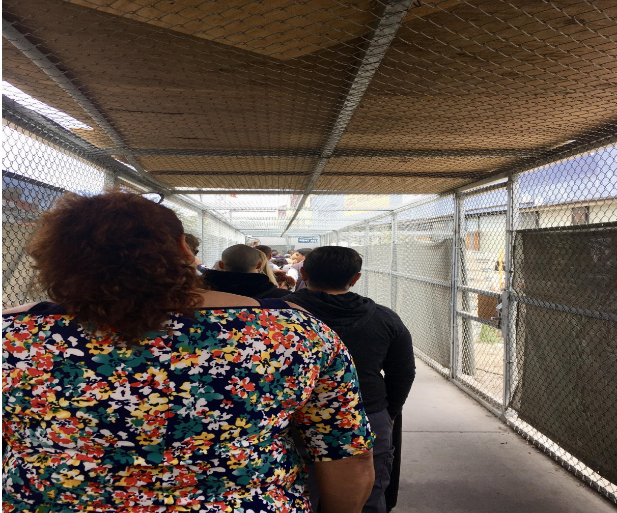
Figure 3.5 DHS cage around pedestrian border crossers at the SYPoE, while undergoing renovations and security enhancements.
