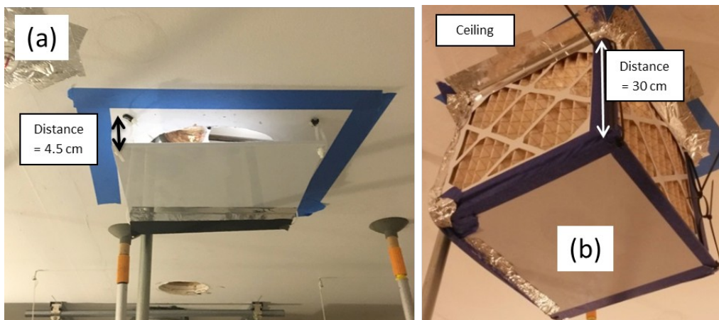
Figure 7. Detail of air inlet: (a) old version; (b) new version (with a ceiling diffuser and MERV 11 air filters)
