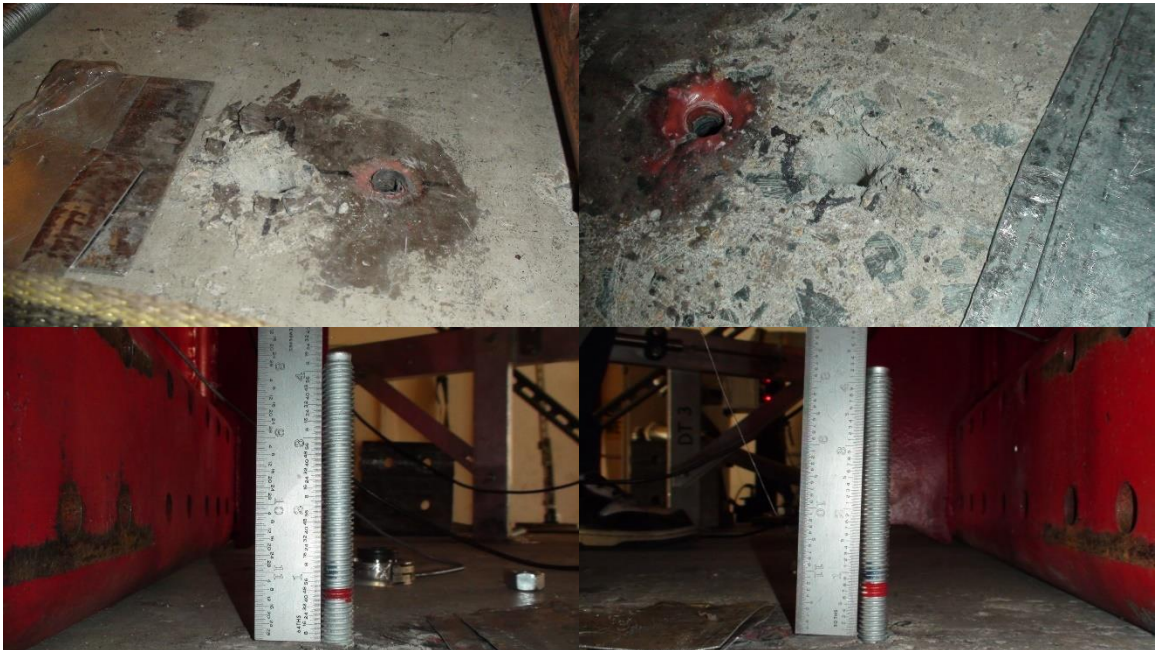
Figure 4-18: N5 Failure Photographs for A1 Anchor Concrete Surface (top left), A2 Anchor Concrete Surface (top right), A3 Anchor No Pullout (bottom left) and A4 Anchor No Pullout (bottom right) for BBM Test Sequence
