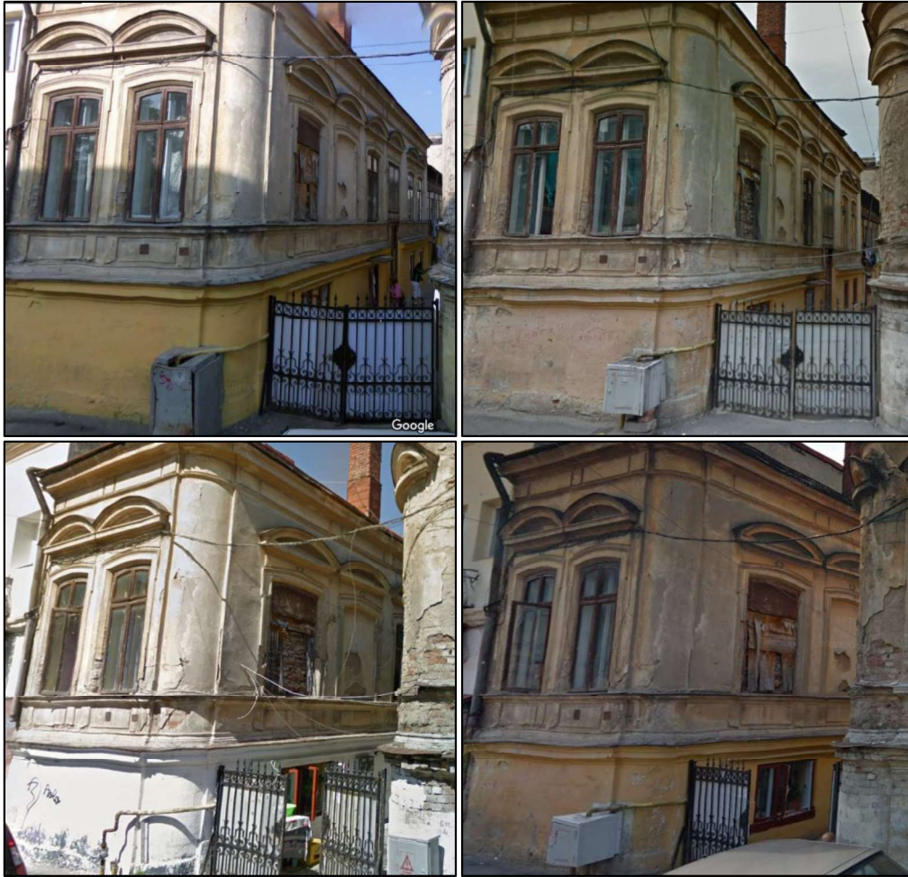
Figure 14: Visual example of informal occupants applying fresh paint to exterior walls; Google Street View images from 2008, 2011, 2014, and 2018 (counter-clockwise).
