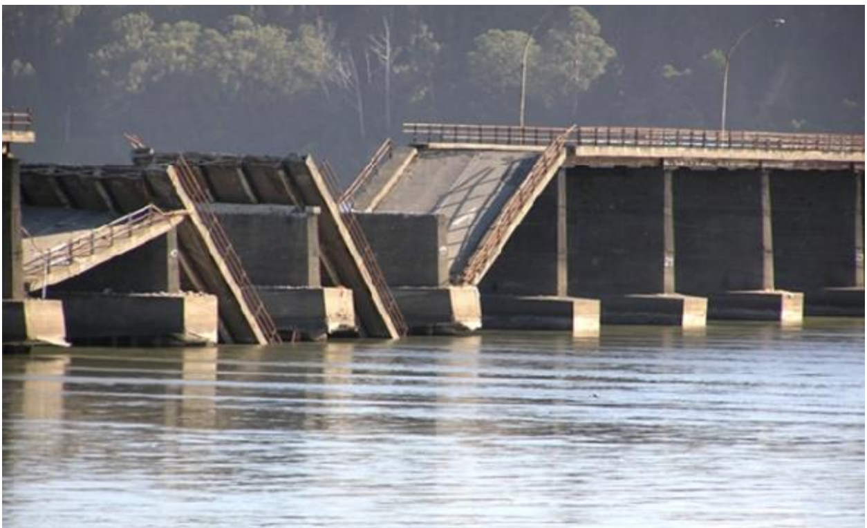
(b) Lateral Unseating of the Puente Bio Bio bridge in Concepción in the 2010 Chile earthquake.
