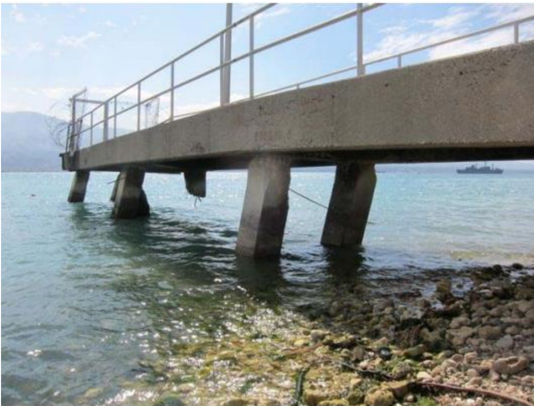
(b) Lateral spreading induced damage to a wharf during the 2010 Haiti earthquake
