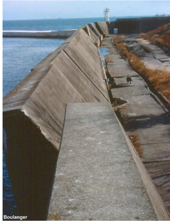
(a) Lateral spreading induced damage to a quay wall after the 1995 Kobe earthquake
