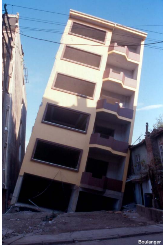
(a) Tilted buildings in Adazapari, Turkey following the 1999 Kocaeli (Turkey) earthquake
