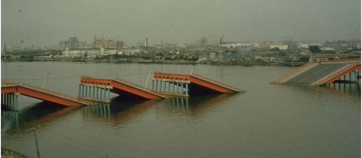
(a) Lateral spreading induced failure of the Showa bridge (lateral soil movement).
