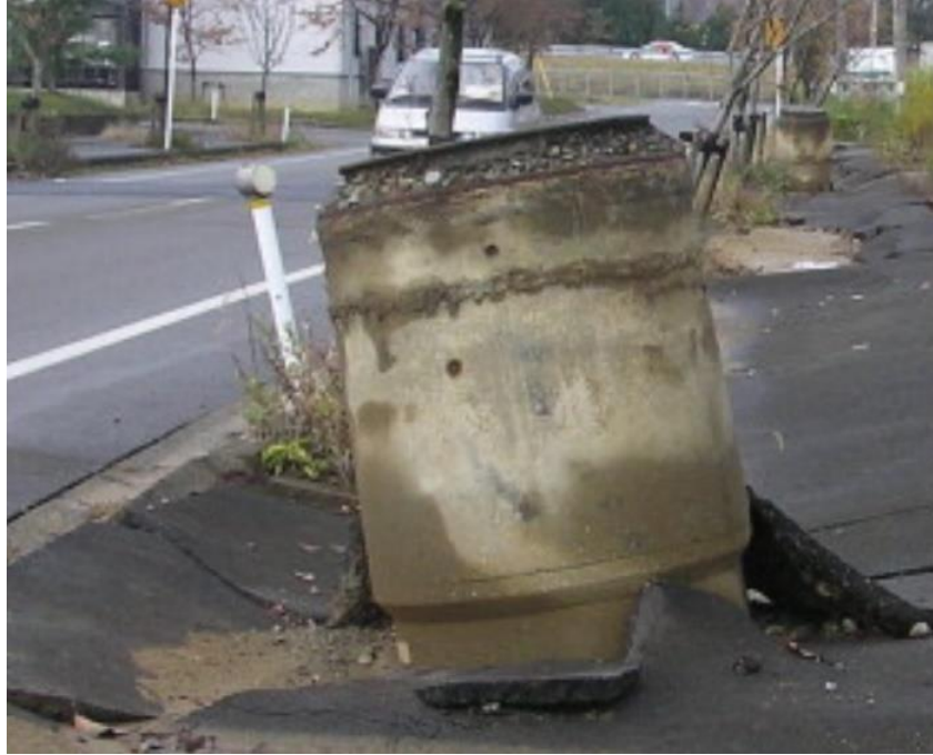
(a) Buoyant rise of an underground utility access hole from the 2004 Niigata Ken-Chuetsu (Japan) earthquake
