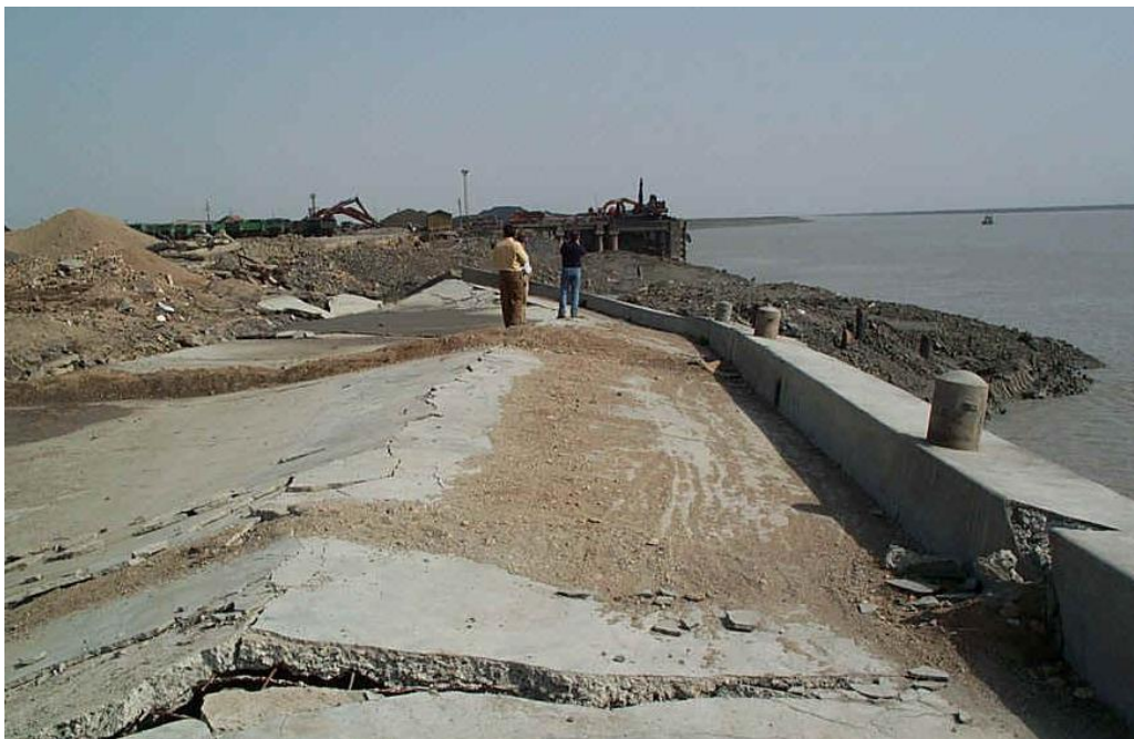
(b) Damages to a quay wall during the 2001 Bhuj Earthquake
