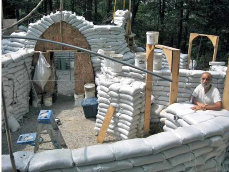
Figure 7.6. An “earth ship,” a home built of sandbags tamped into place, which are then plastered. Gorgeous, energy efficient – and demanding a huge amount of labor.
