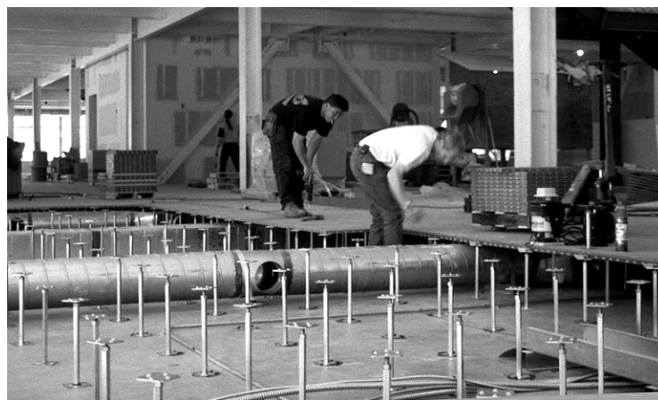
Figure 1 Raised floor installation, above ductwork and cabling in place. (Image: D. Lehrer)
