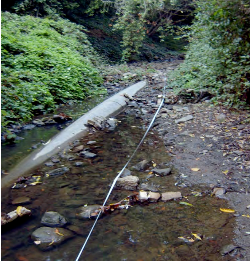
Sewer Line in Bottom of Channel
